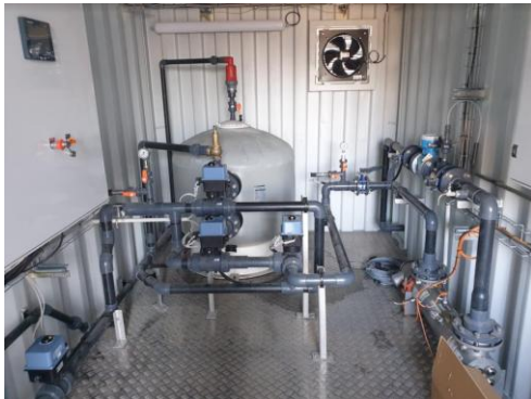
Filtration + UV + Chloration
